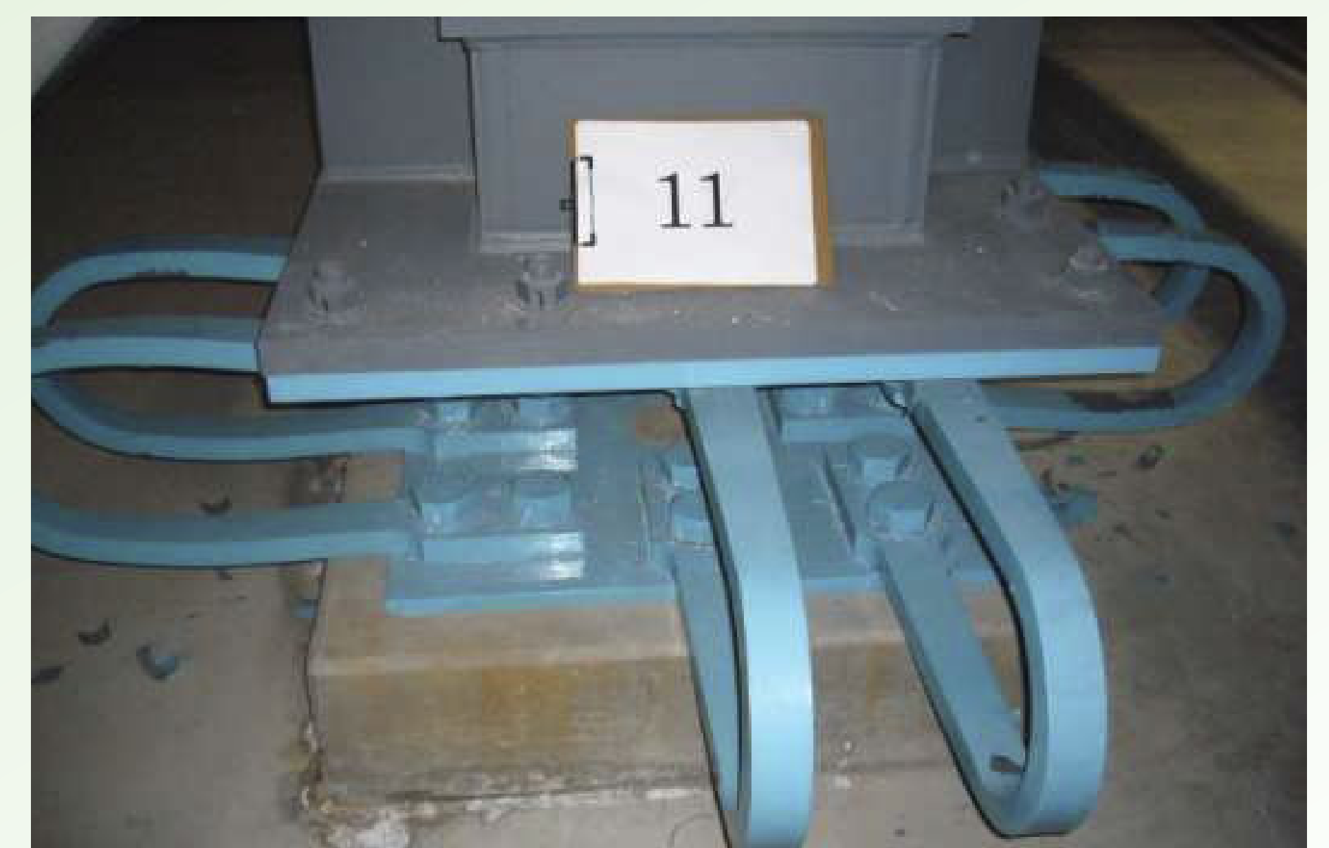
▲ Many ductile steel dampers dissipated earthquake energy
