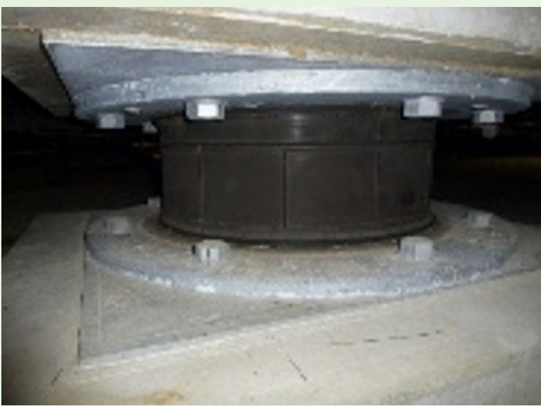
Natural rubber bearing and LRB were used. The bearings remained intact even after 46cm deformation (shear strain of 330%)
